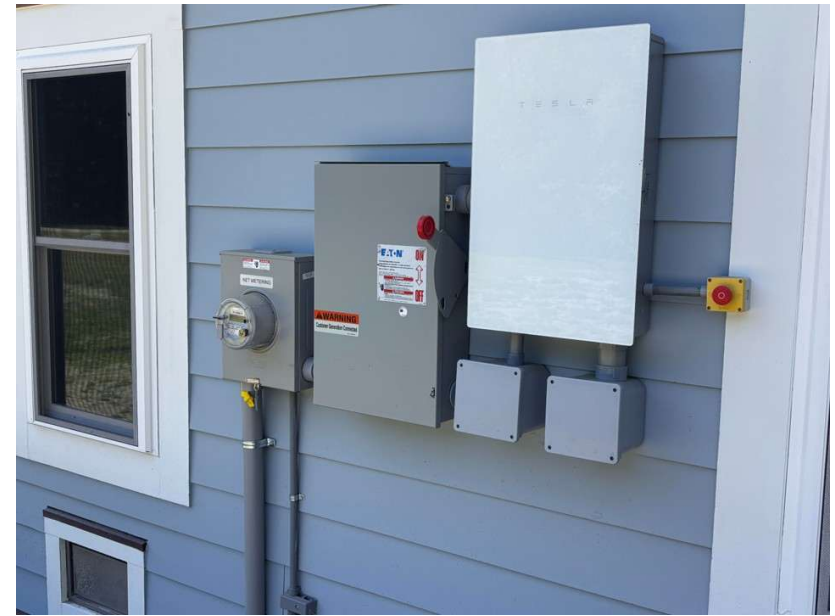
Grid meter, Eaton disconnect switch, and Tesla Backup Gateway
